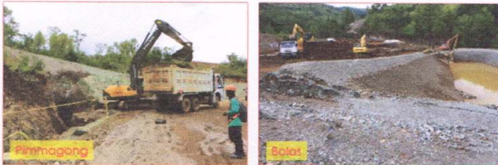
Regular desilting of silt trap (left) and silt pond (right), as one of the maintenance activities for siltation mitigating structures. Collected silt are brought to rehabilitation areas and used as top soil.
