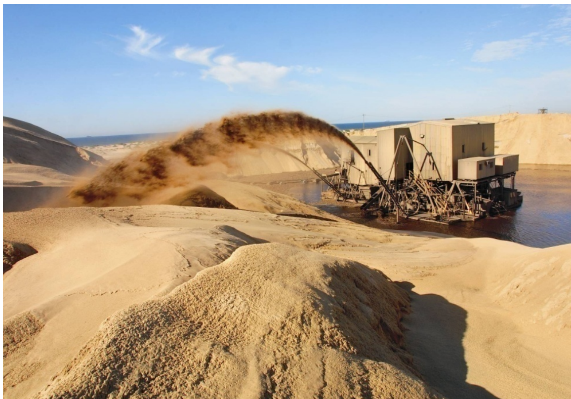
Figure 4.3 Typical Dredge Pond and Concentrator Plant
