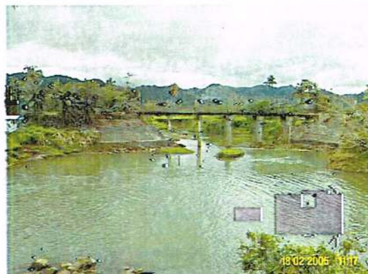
Photo 3-30. Access to Brgys. Siana and Dayano is through this dilapidated bridge from Brgy. Magpayang. The river channel is wide in this section.
