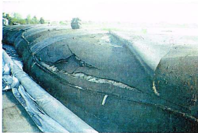
Photo 5-6. After filling, a dry filter cake of mine waste remains (J.R. Wynn).
