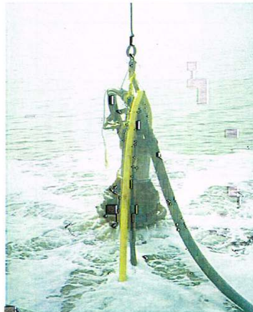
Photo 5-2. The geotextile tubes are fed water by a submersible pump (J.R. Wynn).
