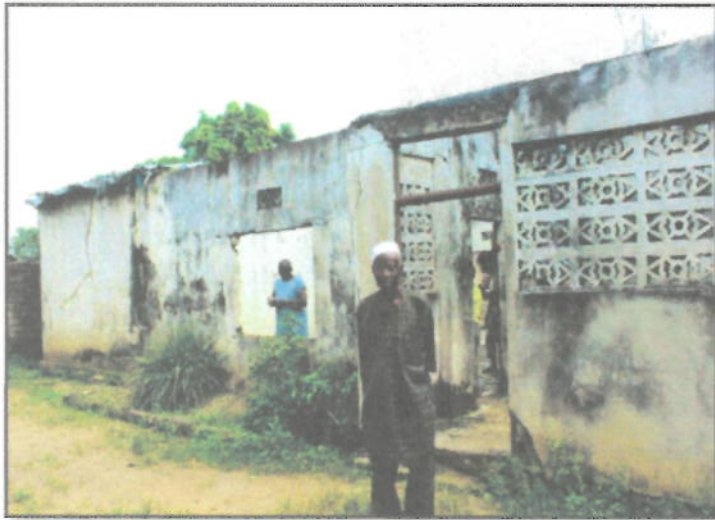
Photo 2: Burnt down house in the Kono District
