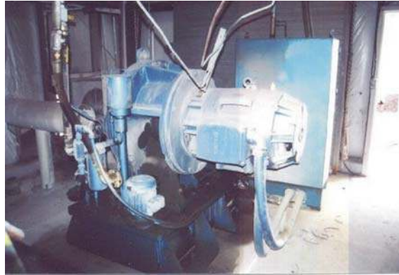
Photo 3-26. A cyanide SO 2 -air detoxification circuit (AM King Industries, Inc.)
