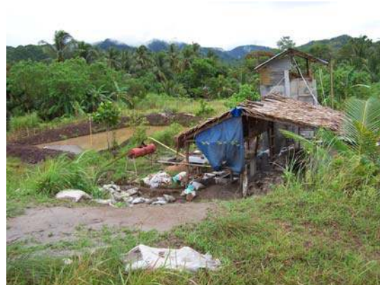
Photo 4-2. The gold CIL plant southeast of Tailings dam 3.
