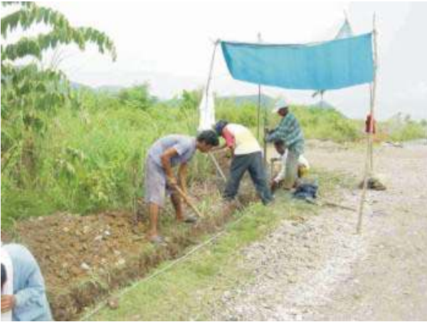
Photo 3-5. Residents of the impact barangays dig the trench for the water distribution pipeline donated by GRC.
