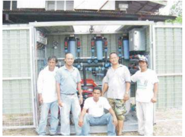
Photo 3-8. The potable water treatment plant donated by GRC to the three (3) direct impact barangays.
